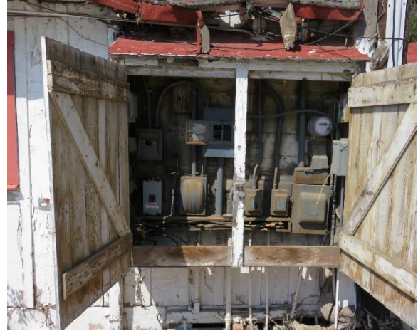
Figure 91. Wooden electrical cabinet interior.
