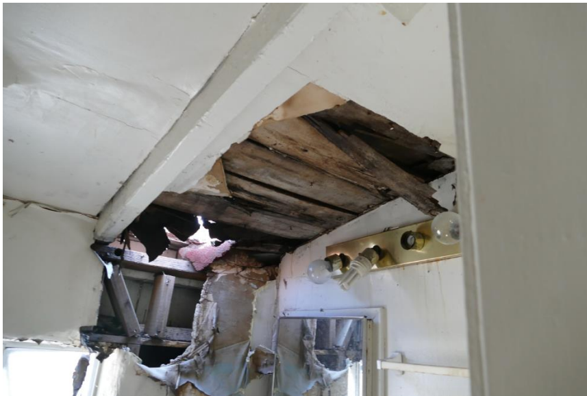
Figure 68. Typical damage to wood framing and finishes resulting from a roof leak at Unit 8. Photo taken facing east.
