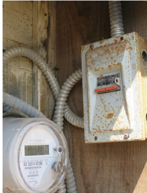
Figure 100. Circuit breaker enclosure (2) 20 amp.
