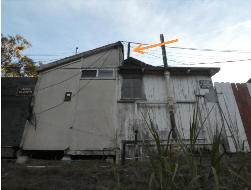
Figure 53. Typical roof form of typical Courtyard North unit. Orange arrow indicates location of clerestory window, shown in Figure 54. Photo taken facing southwest at Unit 28.
