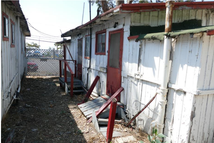
Figure 37. Wood framed entry decks at the South Row West group (steps at Units 3 & 4 used as an example). Photo taken facing south.
