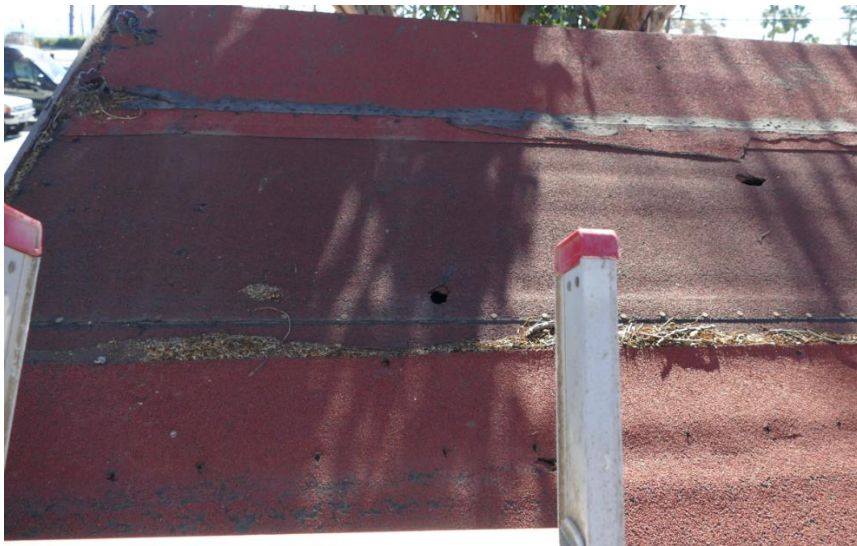
Figure 70. Weathered roofing with open holes and tears susceptible to admitting water directly into the building at Unit 11. Photo taken facing southeast.
