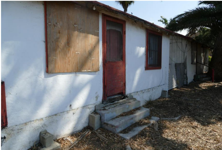
Figure 74. Typical stucco cladding with limited cracks. Photo taken facing northeast at Unit 14.
