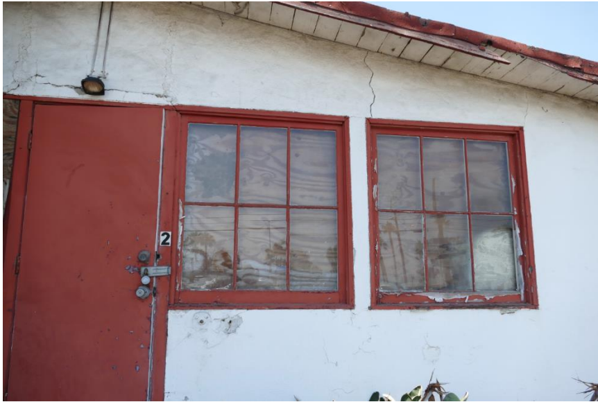
Figure 75. Typical cracks in stucco cladding. Photo taken facing north at Unit 2.
