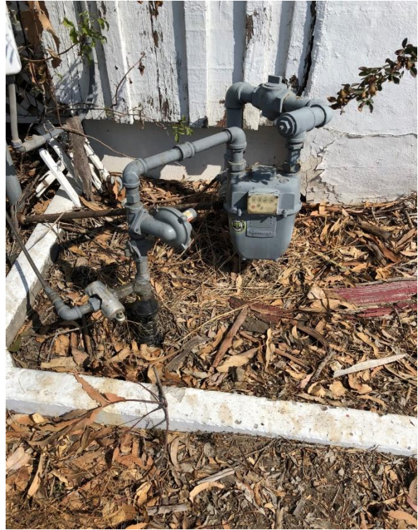
Figure 85. Natural gas meter.
