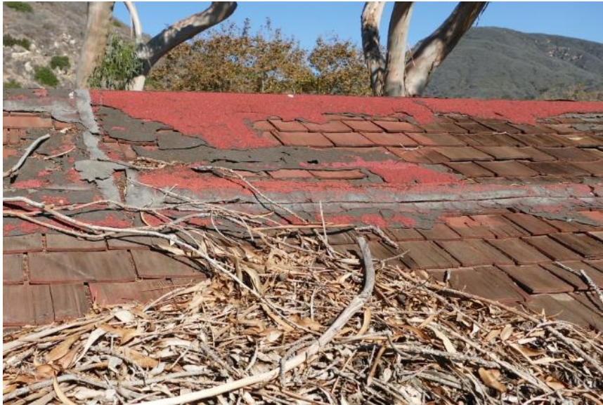
Figure 55. Original wood shakes beneath red asphaltic sheet roofing at Unit 12. Photo taken facing north.
