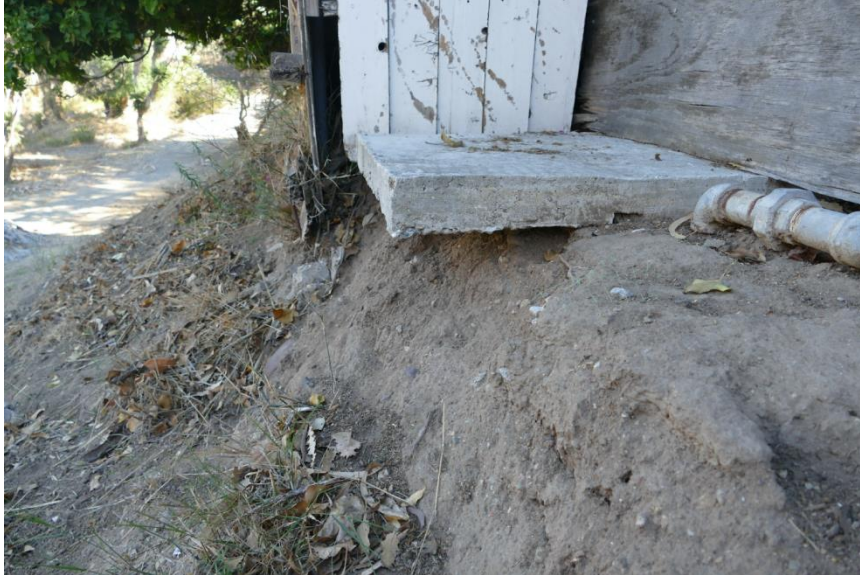
Figure 17. Northeastern embankment failure, undermining a slab on ground. Photo taken facing southeast.
