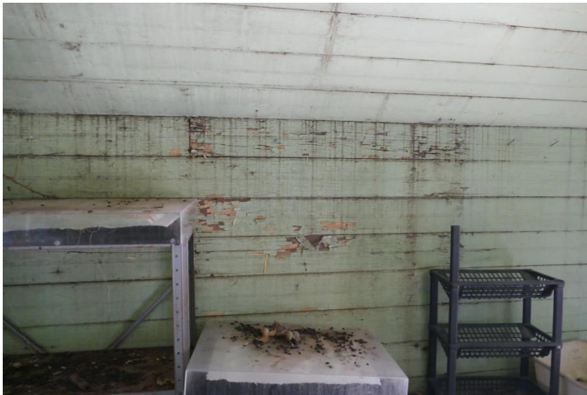
Figure 50. Beaded tongue-and-groove board used as the Storage Shed's walls and ceiling finishes. Photo taken facing southeast.
