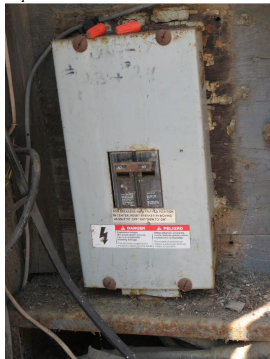
Figure 102. Circuit breaker enclosure (1) 60 amp.
