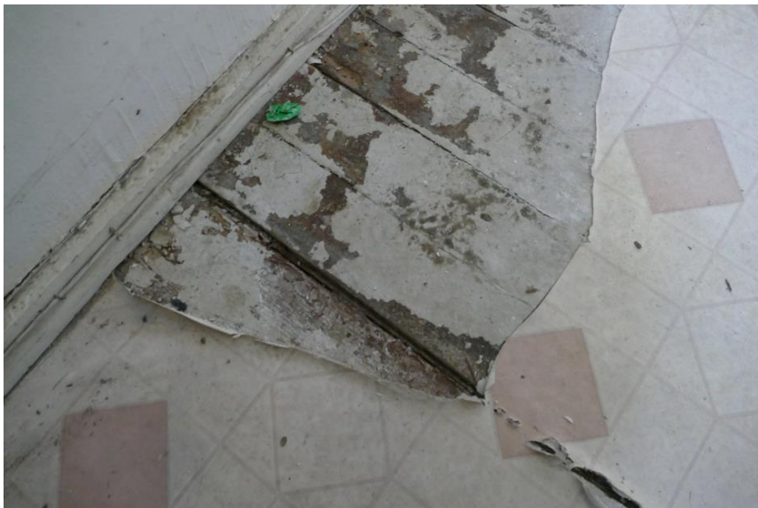
Figure 66. Original 1x4 tongue-and-groove floor decking with vinyl flooring at the interior of Unit 6. Photo taken facing north.
