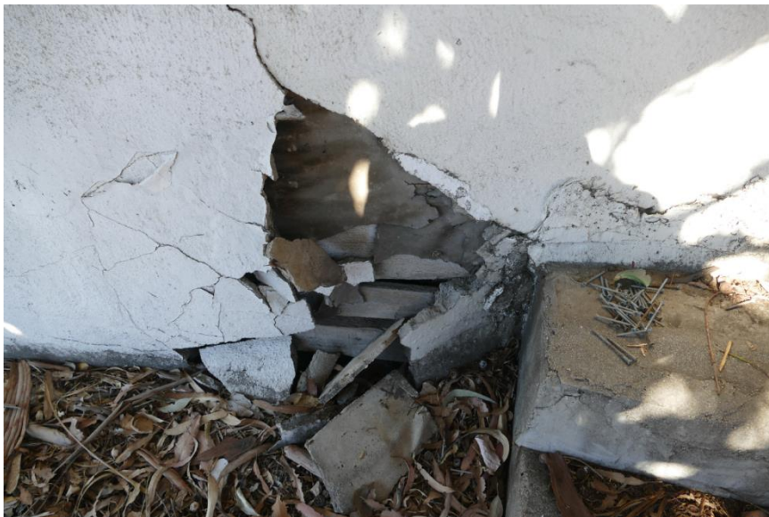
Figure 76. Damaged stucco cladding next to the entry stairs of Unit 15. Photo taken facing northwest.
