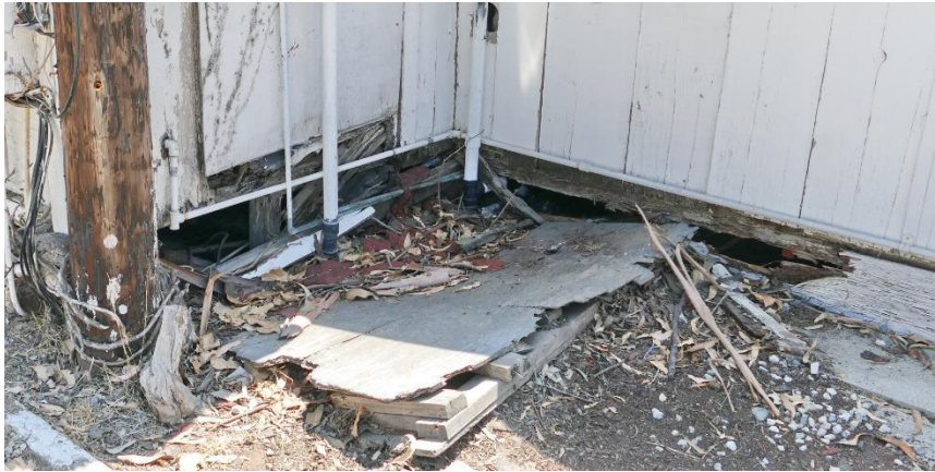
Figure 73. Deteriorated wood cladding in proximity to soil at Units 7 and 8. Photo taken facing south.
