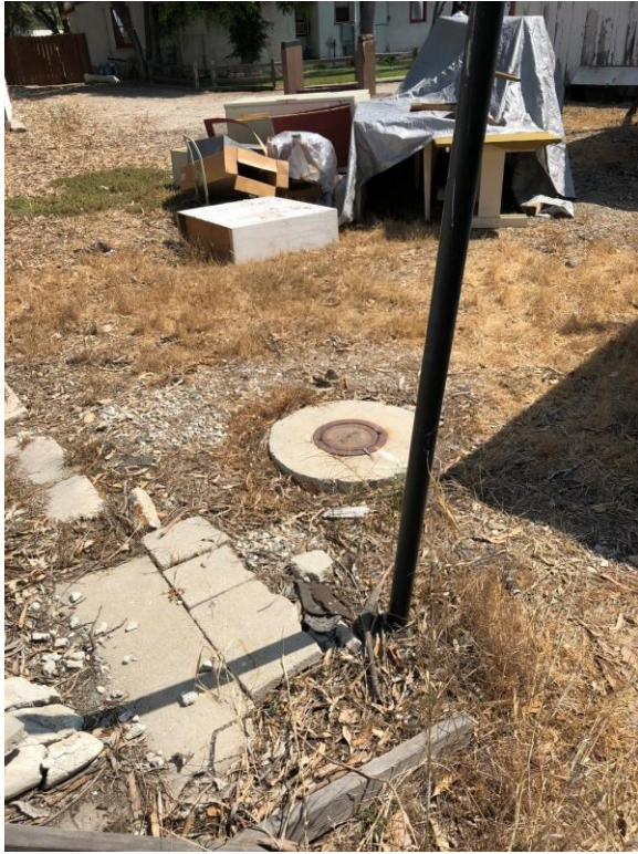
Figure 88. Sewer storage (septic) tank.
