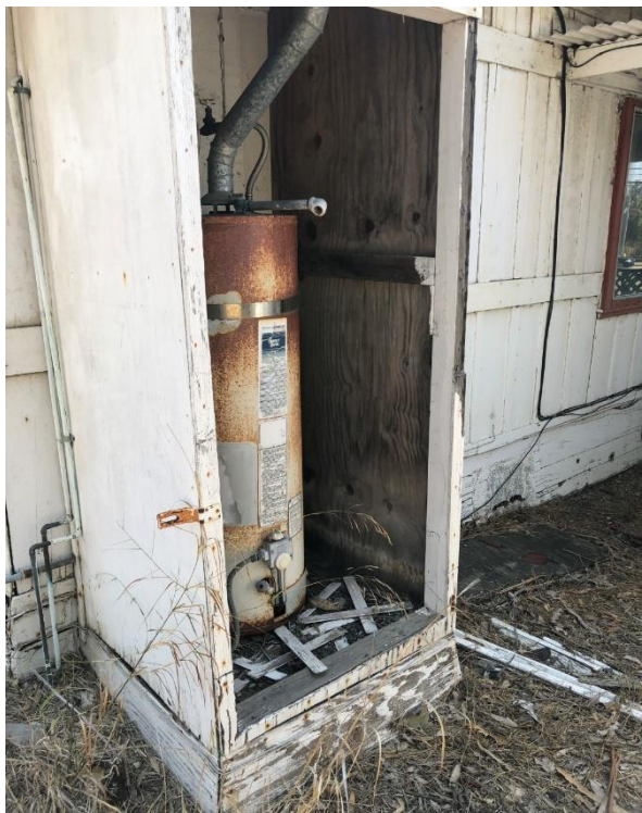
Figure 87. Water heater and enclosure.
