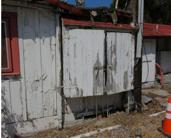
Figure 90. Wooden electrical cabinet exterior.
