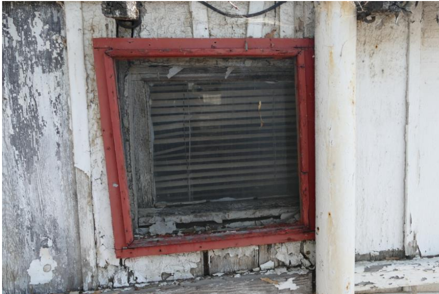
Figure 69. Example of deteriorated wood window. Photo taken facing southeast at Unit 11.
