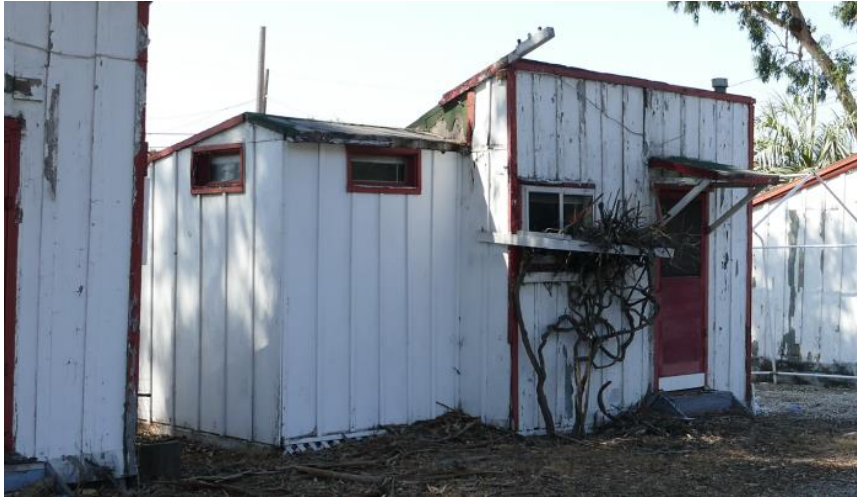
Figure 45. Shed roof addition to the east of Unit 18. Photo taken facing southwest.
