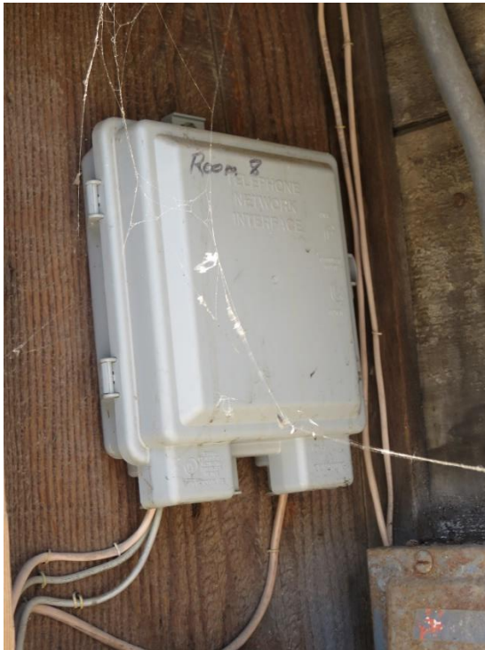
Figure 103. Telephone network interface
