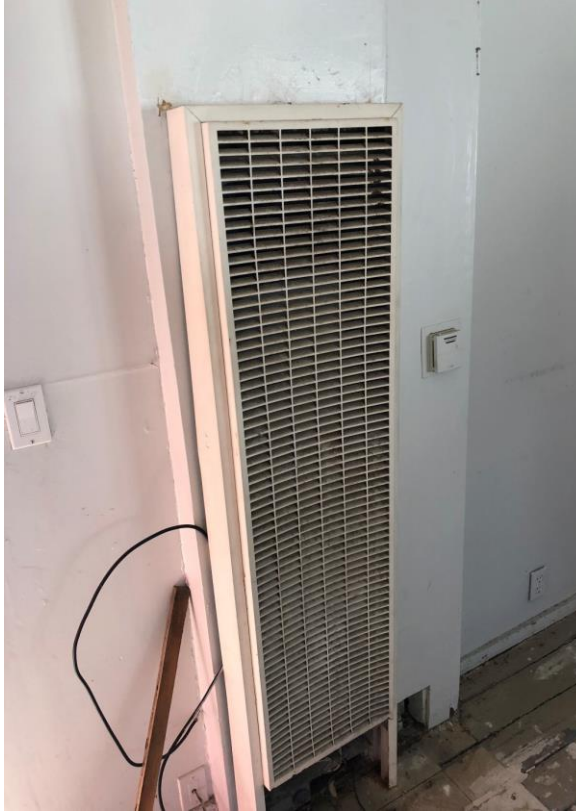
Figure 79. Gas Furnace Interior.
