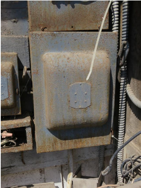
Figure 99. Main disconnect switch.
