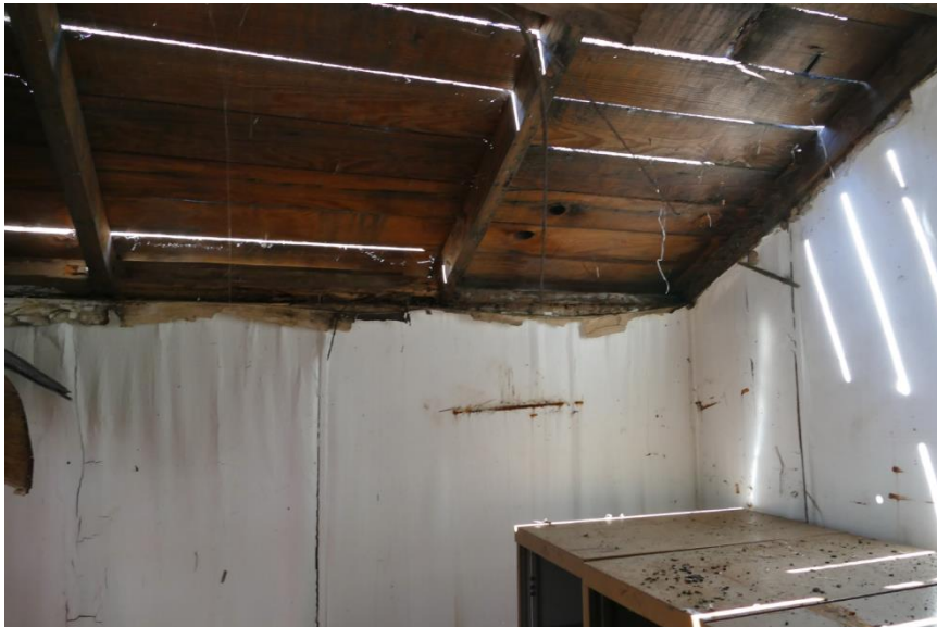
Figure 72. Water intrusion from the exposed roof sheathing into the wall below at Unit 28. Photo taken facing northwest.
