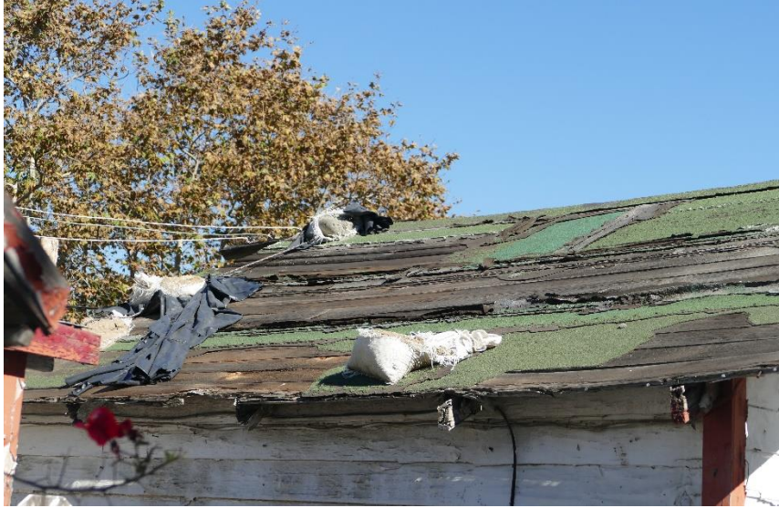
Figure 71. Areas of exposed roof sheathing and heavily deteriorated roofing membrane on the west roof pitch of Unit 28. Photo taken facing northeast.
