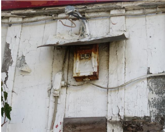
Figure 109. Unit circuit breaker enclosure under shelter.
