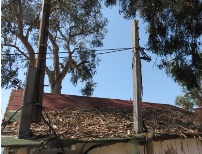
Figure 111. Electrical / Telephone Distribution Pole.
