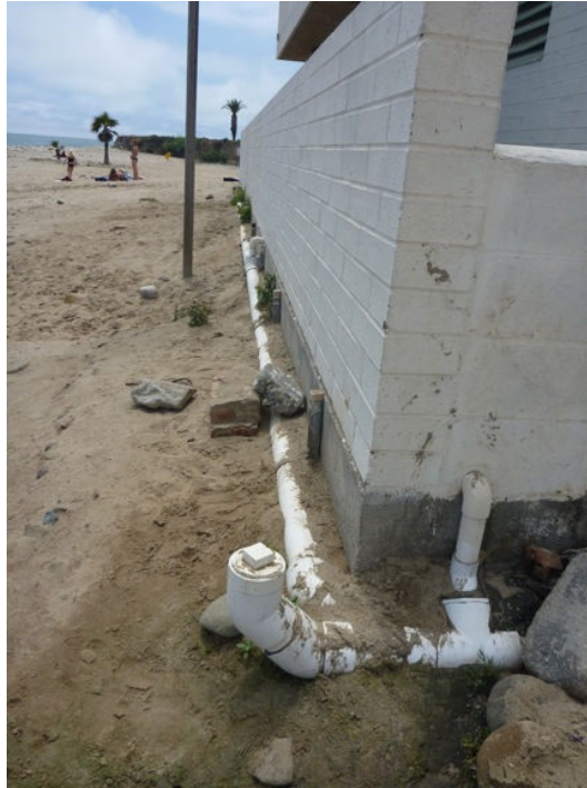
Figure 5-2 Photograph of the collection system at the Topanga Beach Restroom showers
