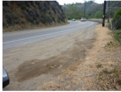
Figure 6-2 RV discharge on shoulder of Topanga Canyon Blvd., May 31, 2013
