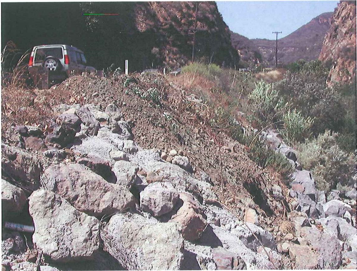
Figure 26 – Soil Berms Sloughing into Creek
