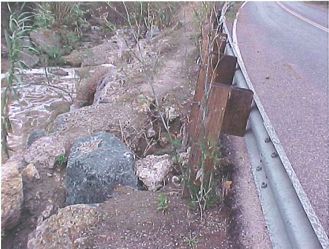
Figure 24 – Erosion Caused by a Fill Slope on SR-27
