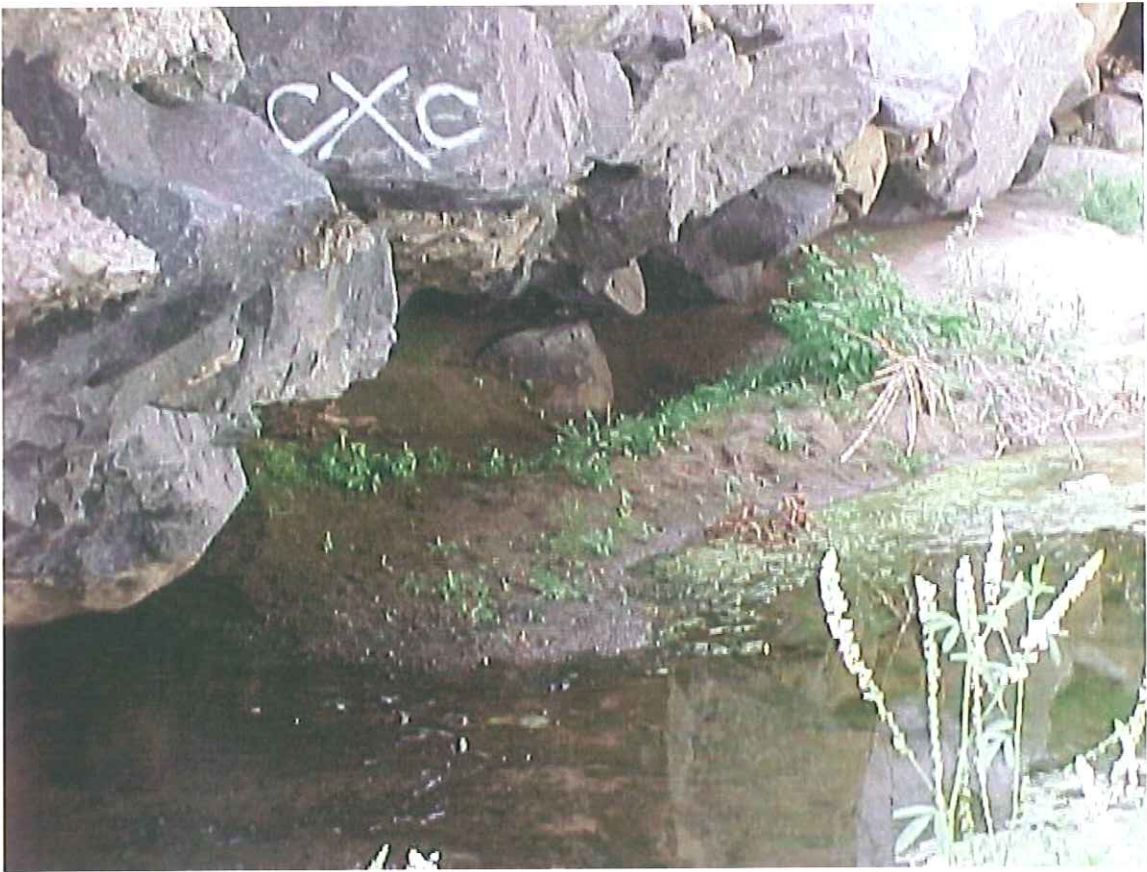
Figure 34 – Undercutting of Riprap near Steelhead Location
