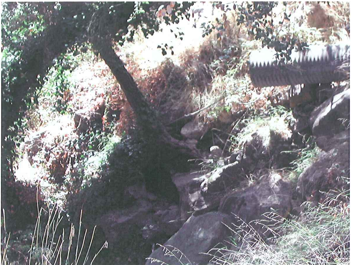
Figure 23 – View of Culvert Causing Erosion
