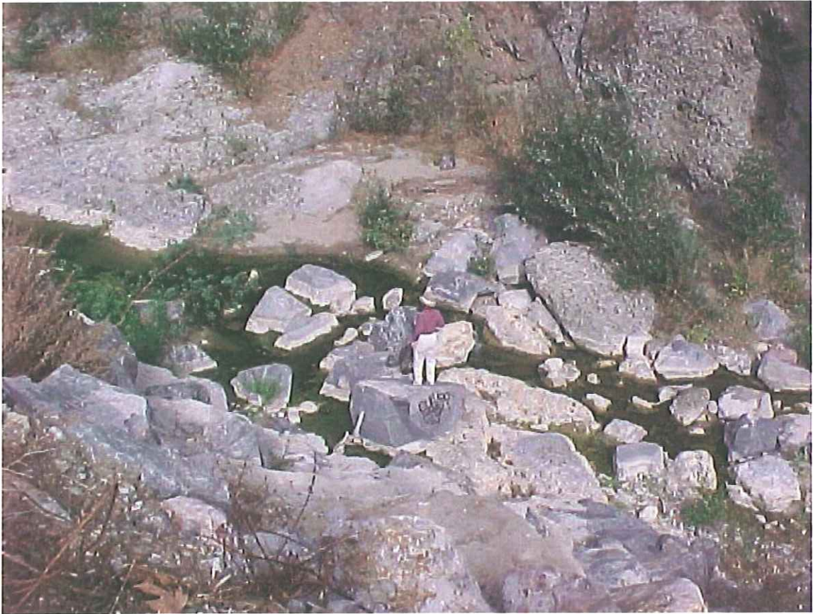
Figure 35 – Loose Boulders in Topanga Creek from Riprap
